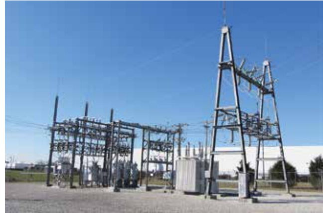
Substations, like the Asahi substation, can be found across South Kentucky RECC's service territory. Photo: East Kentucky Power Cooperative
