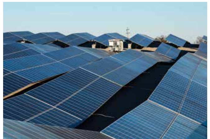
South Kentucky RECC offers solar power to members from its solar farm near Winchester. Photo: Tim Webb
