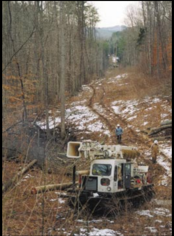
Warren RECC, headquartered in Bowling Green, brought their bucket/digger truck on tracks to aid in restoring power.
