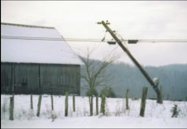
This pole broke, but it didn't fall.
